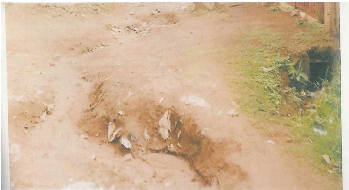
Plate 2: Road network that is almost washed-off by water erosion along the ECWA dispensary road, Koro. The width of the road has become so reduced that is almost impassable for four wheeled vehicles.
