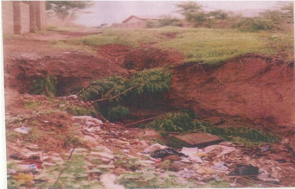
Plate 1: An open space severely affected by gully erosion along Koro grammar School.
